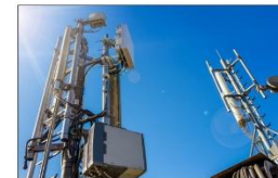
Telecommunication base station
