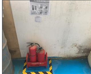
Photo of fire safety equipment Unblocked fire extinguishers and fire extinguishers were placed at the proper height 2.JPG
