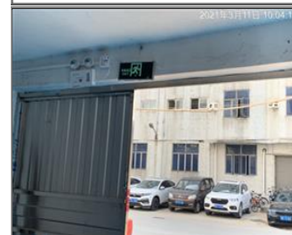
Photo of fire safety equipment Emergency light and lampit exit sign 1 for production building.JPG
