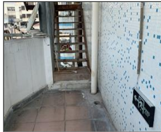
Photo of fire safety equipment Lampit evacuation indication sign 2 for dormitory building.JPG
