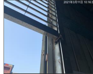
Photo of the inside of the main production hall Fixing device for rolling door.JPG
