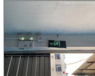
Photo of fire safety equipment Emergency light testing.JPG
