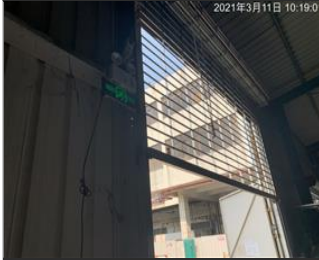
Photo of fire safety equipment Emergency light and lampit exit sign for warehouse building.JPG
