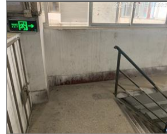
Photo of fire safety equipment Lampit evacuation indication sign 2 for production building.JPG
