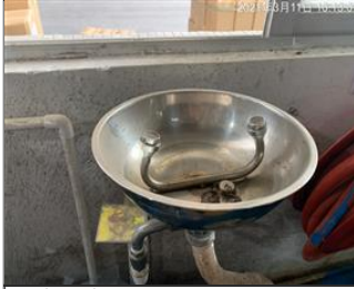
Photo first aid facilities Eye washing station.JPG
