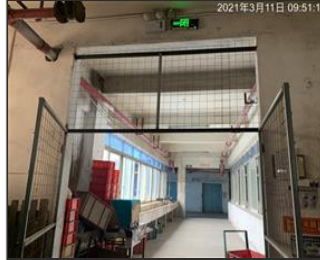
Photo of fire safety equipment Emergency light lampit exit sign and unblocked exit in production building.JPG
