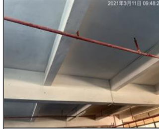
Photo of fire safety equipment Fire sprinkling system.JPG
