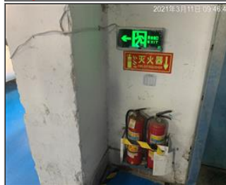
Photo of fire safety equipment Lampit evacuation indication sign 3 for production building and fire extinguisher.JPG
