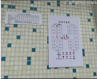
Photo of fire safety equipment Evacuation map in dormitory building.JPG
