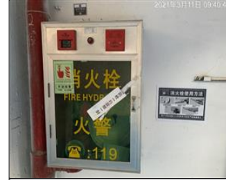
Photo of fire safety equipment Fire hydrant and fire alarm.JPG
