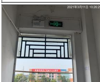
Photo of fire safety equipment Emergency light and lampit exit sign 2 for dormitory building.JPG
