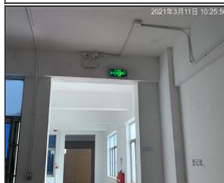
Photo of fire safety equipment Emergency light and lampit exit sign 1 for dormitory building.JPG
