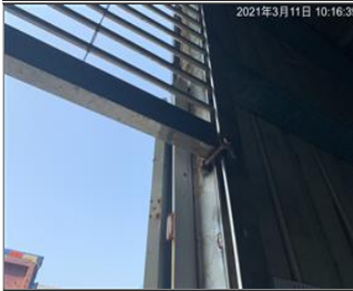
Photo of the inside of the main production hall Fixing device for rolling door.JPG
