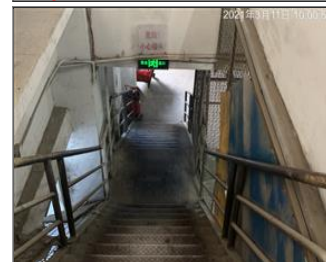
Photo of fire safety equipment Lampit exit sign for production building.JPG
