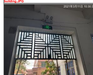
Photo of fire safety equipment Emergency light and lampit exit sign 3 for dormitory building.JPG
