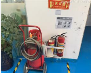
Photo of fire safety equipment Unblocked fire extinguishers and fire hydrant were placed at the proper height 1.JPG
