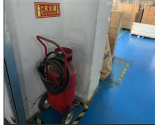
Photo of fire safety equipment Unblocked fire extinguishers.JPG
