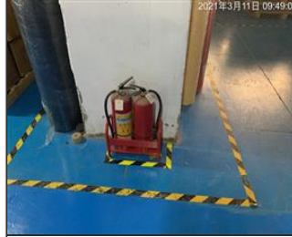
Photo of fire safety equipment Fire extinguishers.JPG
