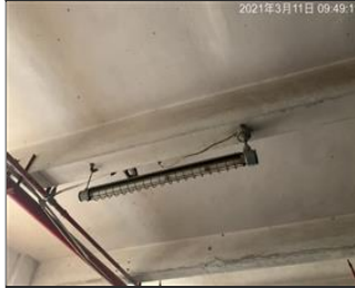
Photo of the inside of the main production hall Explosion proof light.JPG
