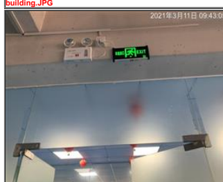
Photo of fire safety equipment Emergency light and lampit exit sign 2 for production building.JPG
