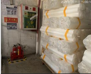
Photo of fire safety equipment Unblocked fire extinguishers and fire hydrant.JPG
