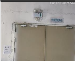
Photo of fire safety equipment Non Exit sign was marked.JPG
