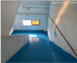
Photo of fire safety equipment Lampit evacuation indication sign 1 for production building.JPG
