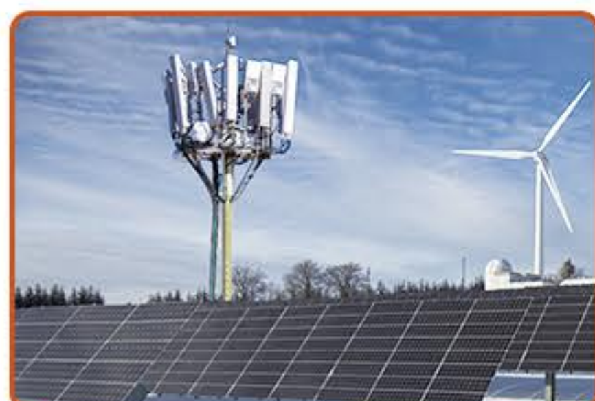
COMMUNICATION BASE STATION
