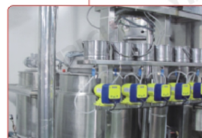
FCA: In-line flavor, color, acid dosing and mixing system 色香酸的在线自动加注混合系统
