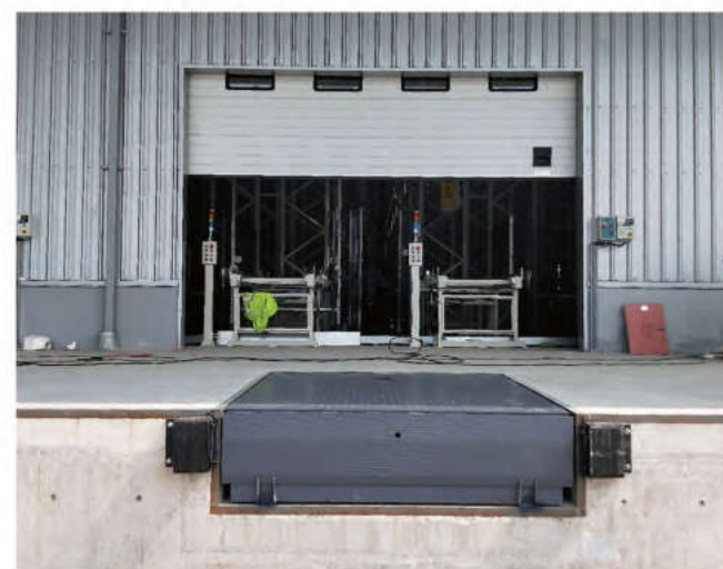
装卸平台 Loading and unloading platform
