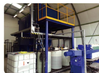
Water treatment system
