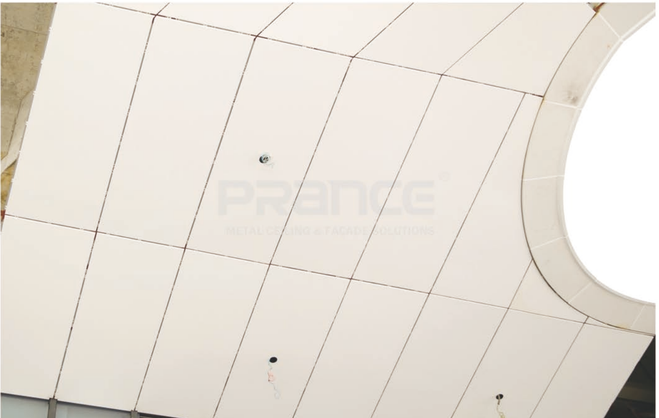
▲ Metal Flat Panel Ceiling
